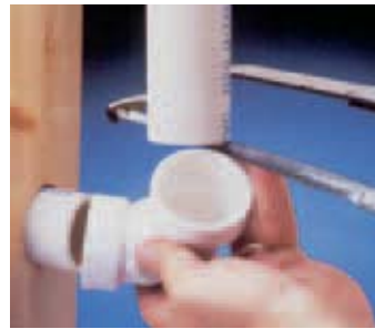
Damaged or leaking fitting is cut out
